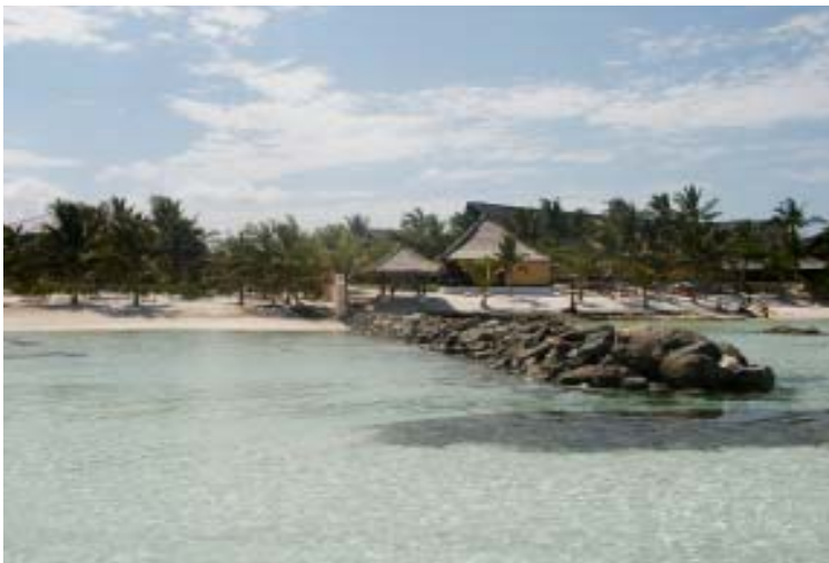
The placement of concrete stabilization structures and the conclusion of the groin structure was recommended to allow for sand nourishment.
